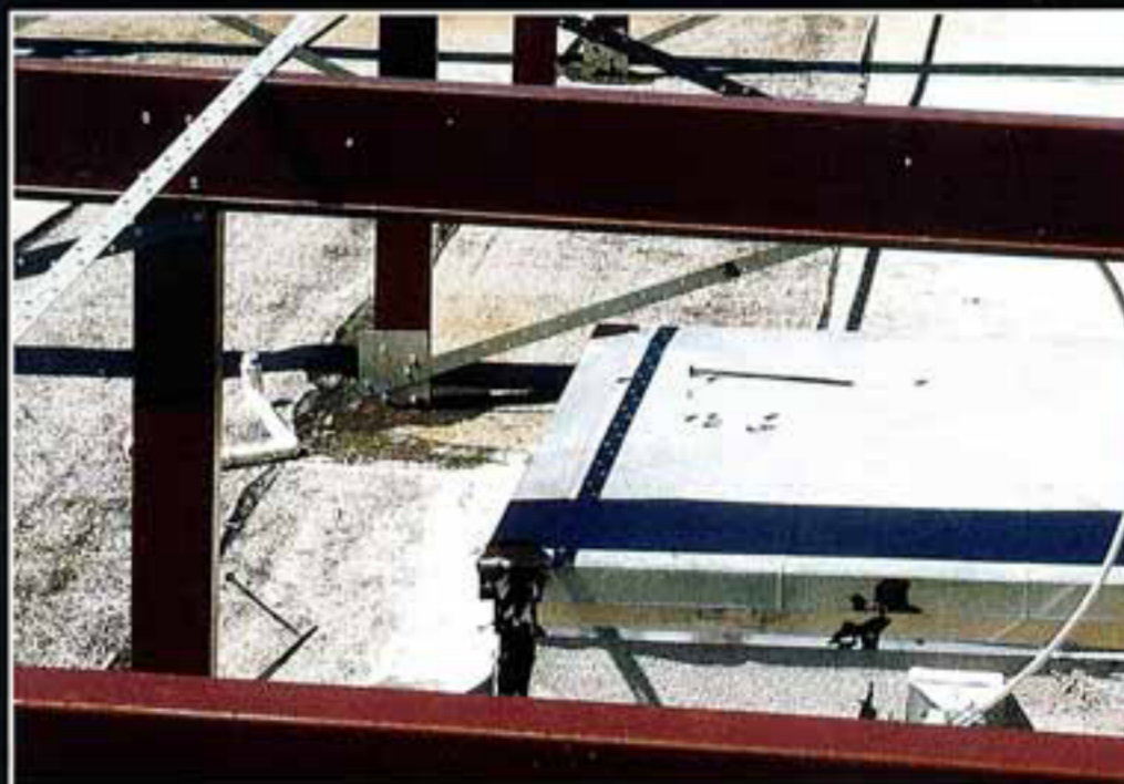
Initial steps for a Galvalume metal roof conversion of a flat roof. p. 14
