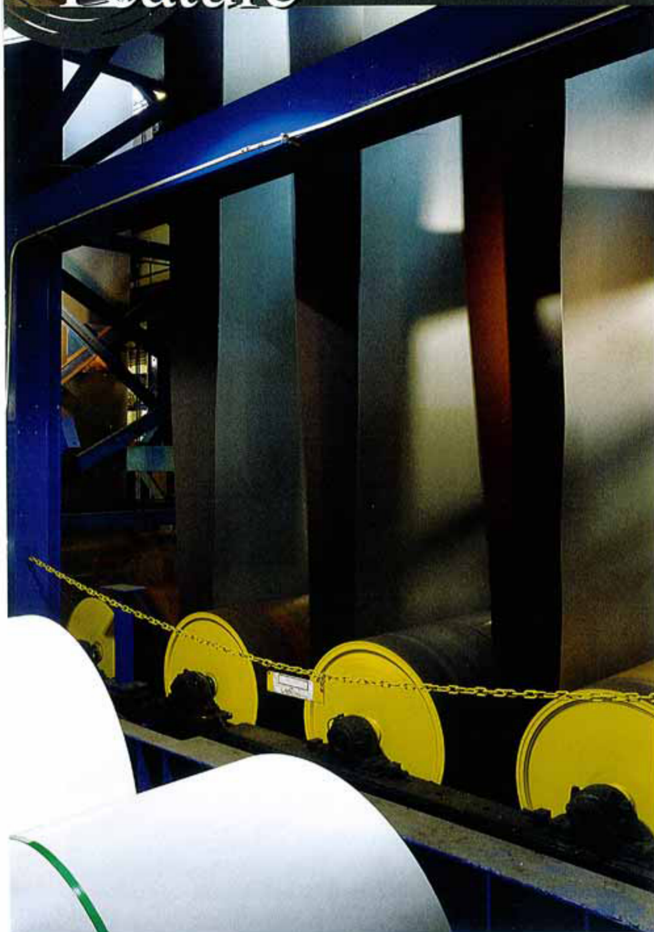
As part of Centria's Ambridge facility retrofit project was the upgrade of its accumulator tower.
